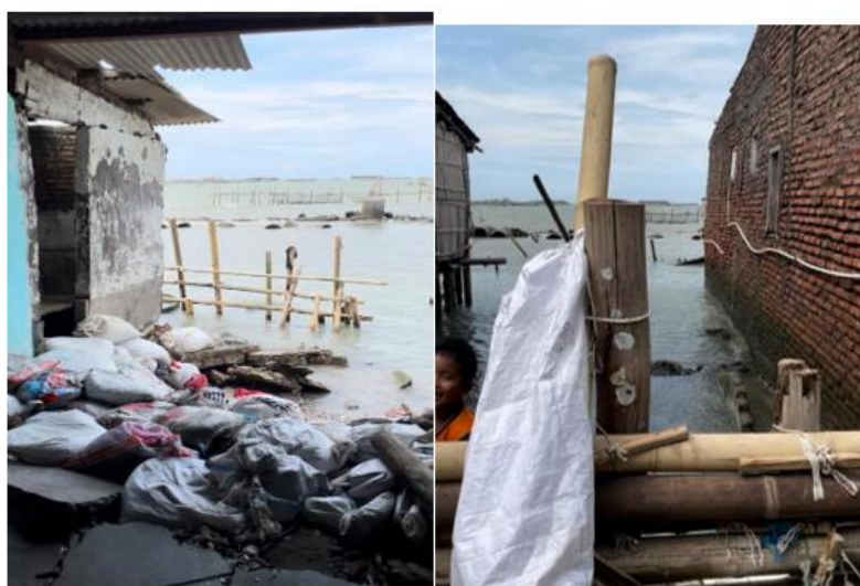
Fig.2 The condition of a Tambak Lorok resident's house severely damaged by flooding, with cracked walls and a damaged roof. Source: (Field documentation, June 2024).
